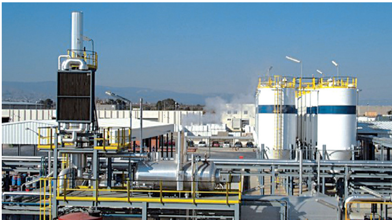
Trisa industrial waste treatment and recovery plant. Constanti. Tarragona
